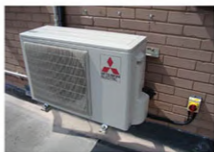
Good ventilation for outdoor location
