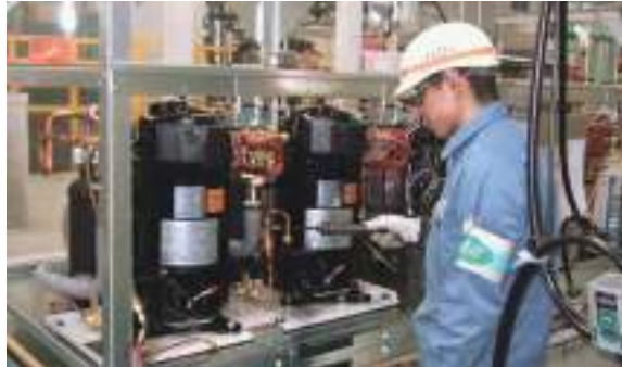
Compressor also developed and manufactured by Mitsubishi Electric* Refrigerant leak inspection process using helium gas
